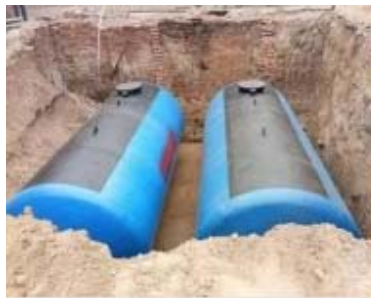
Buried Oil Tank
