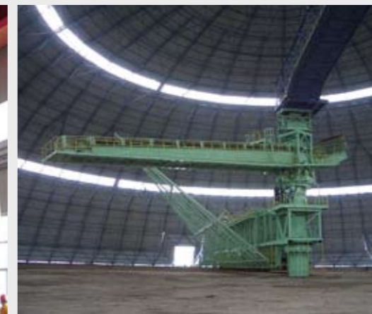
堆取料机 Stacker and reclaimer
