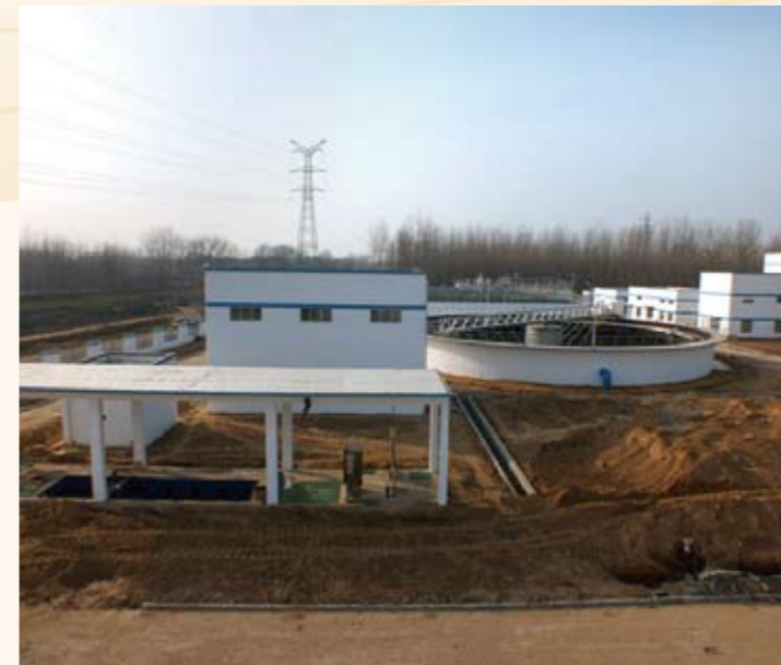
江苏宿迁城北污水处理厂一期工程 Jiangsu Suqian Chengbei Wastewater Treatment Plant Project (Phase I)
